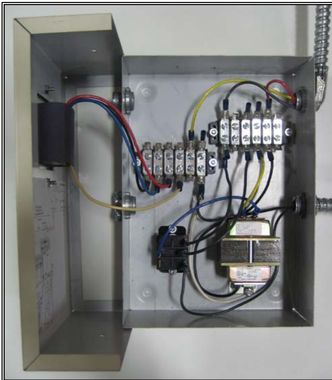
Figure 4: Control Box for Forced Air Draft
